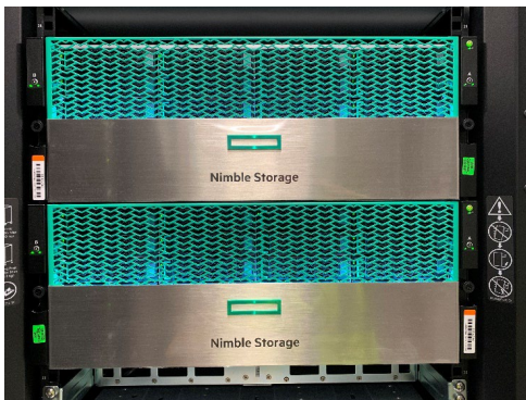
Accelerator Cluster disk storage – two HPE nimble storage chassis
