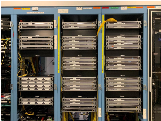
Fiber shelves in APS datacenter for accelerator, beamlines, LOMs
