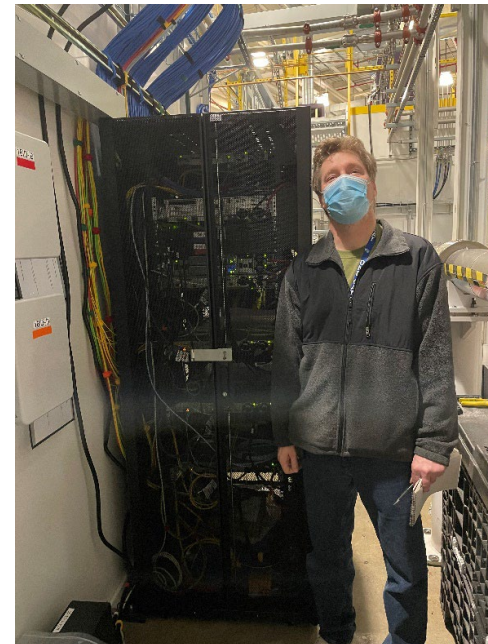
S16 network isolation boxes
