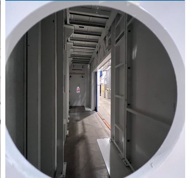
11-ID shielded enclosure
